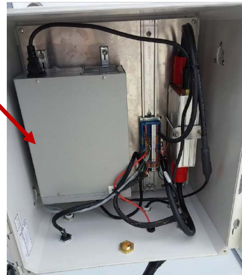
Power supply and SAS deck unit
