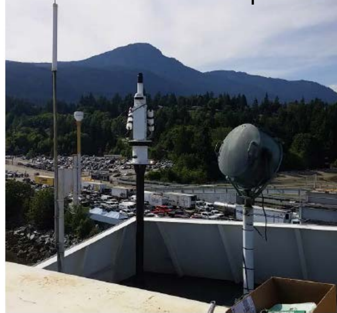
SAS ST mounted on a pedestal
